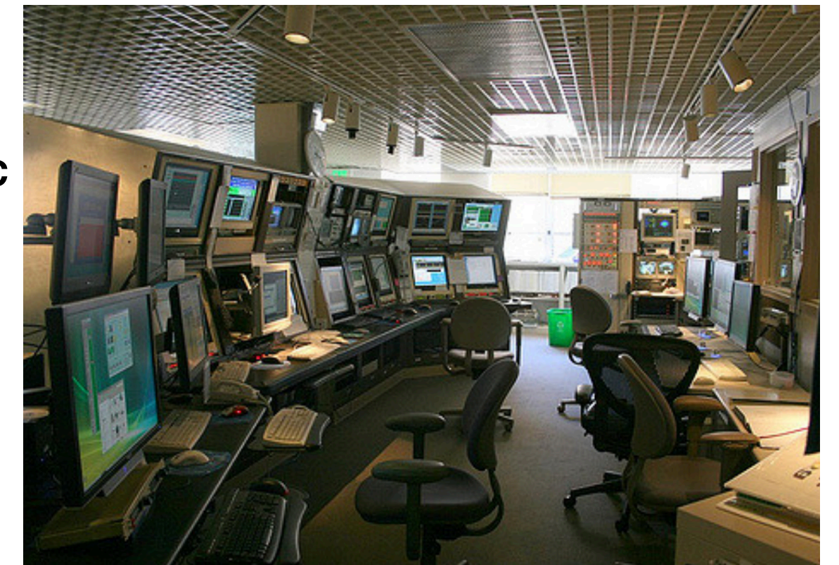
High level controls
